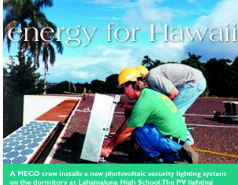
A MECO crew installs a new photovoltaic security lighting system on the dormitory at Lahainaluna High School. The PV lighting system was paid for through MECO's Sun Power for Schools program.
