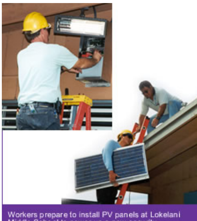
Workers prepare to install PV panels at Lokelani Middle School to power up a new security lighting system.
