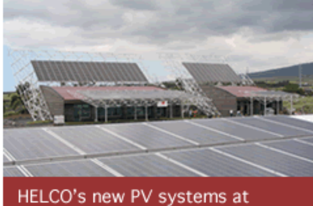
HELCO's new PV systems at NELHA's Hawaii Gateway Energy Center demonstrate the use of renewable technology.
