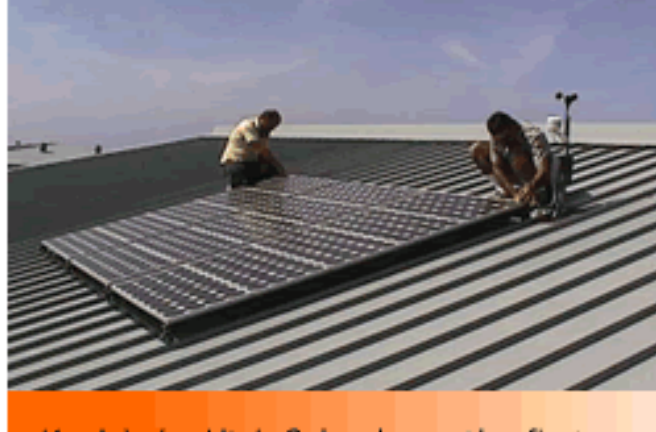
Kealakehe High School was the first Big Island school to receive a photovoltaic electric system, installed in July, 1998.
