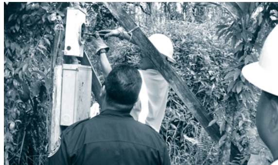
A HELCO lineman safely removes a tampering device at a residence as a Hawaii Police Department officer and a HELCO safety administrator secure the premises.
