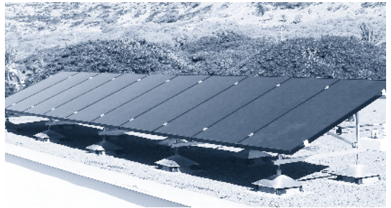
These photovoltaic panels atop Waianae Intermediate School are part of a two-kilowatt solar electric system installed in December 2006, through the Sun Power for Schools program.
