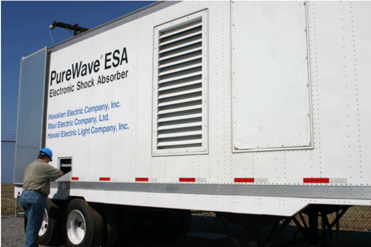
Electronic Shock Absorber at Lalamilo Wind Farm site.
