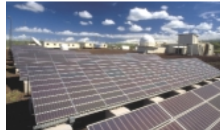
Photovoltaic facility in Kihei, Maui
