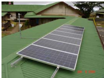
Naalehu School, 1 kilowatt
