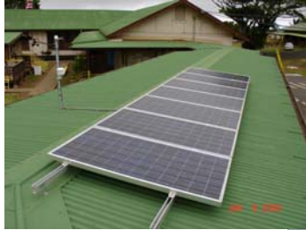
Naalehu School, 1 kilowatt
