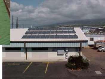
HELCO Kona Baseyard, 5 kilowatts
