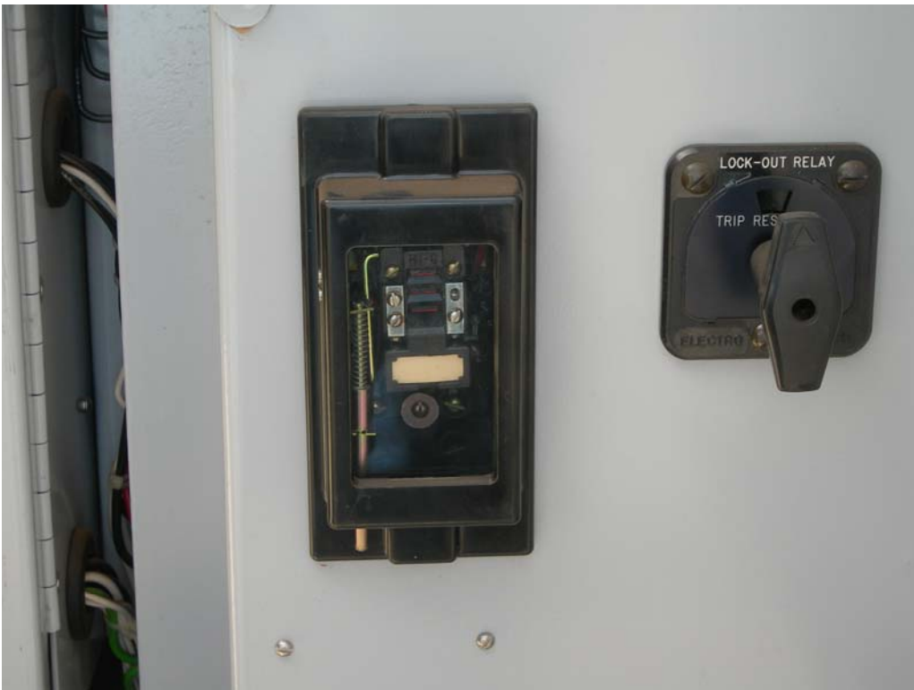
Figure 7: Transformer Fault Pressure Target Relay and 86T Lockout Relay
