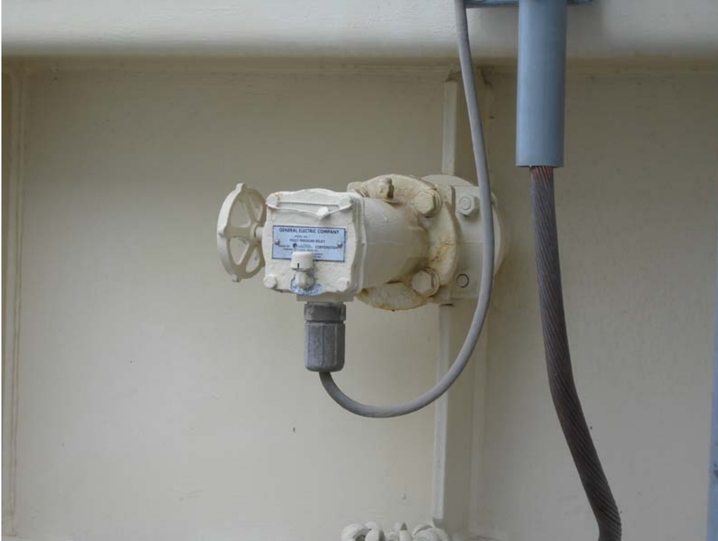
Figure 6: Transformer Fault Pressure Sensor Qualitrol.
