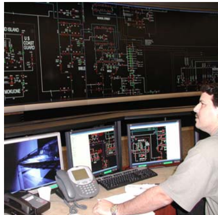
HECO recently upgraded its Energy Management System, the "brain" that controls the electric system.
