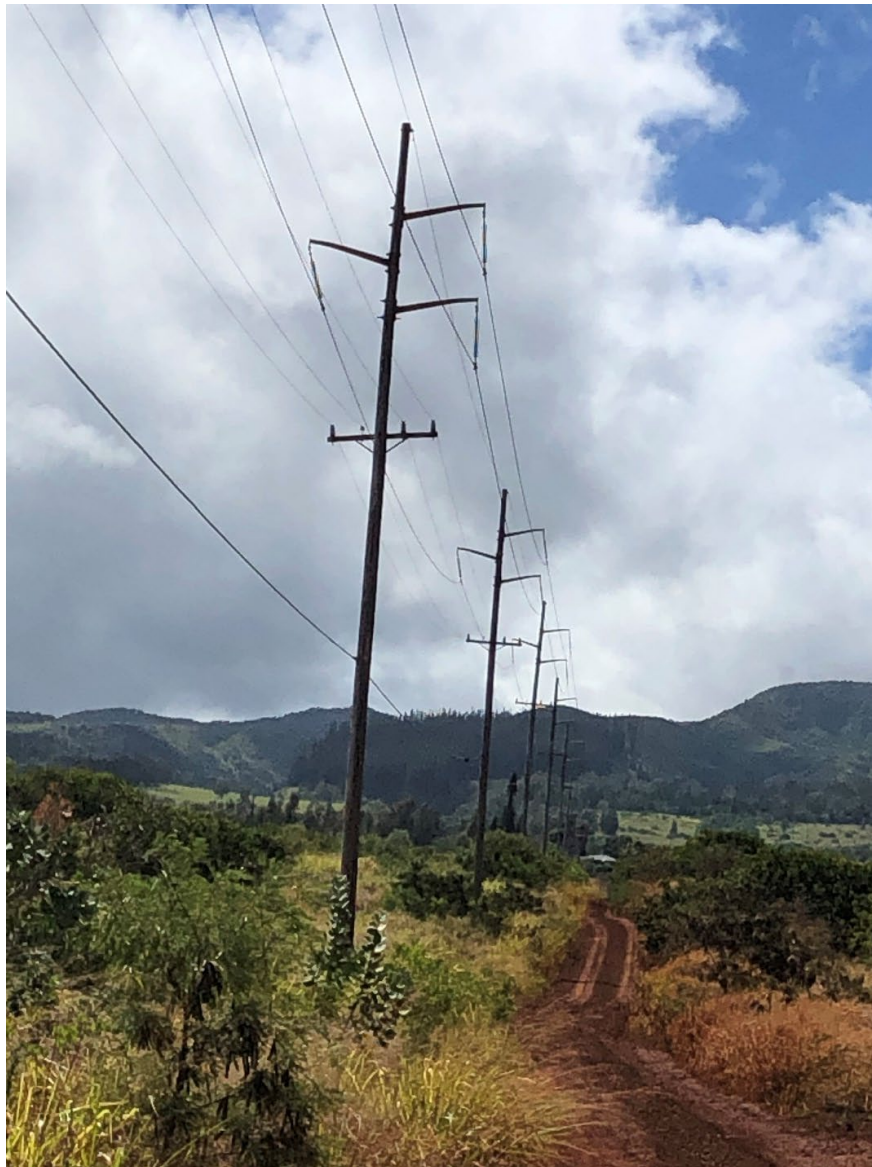
Figure 8 – Lahaina #2 Mauka 69kV Circuit and 1381 12kV Circuit, Kapalua, Maui 2020.
