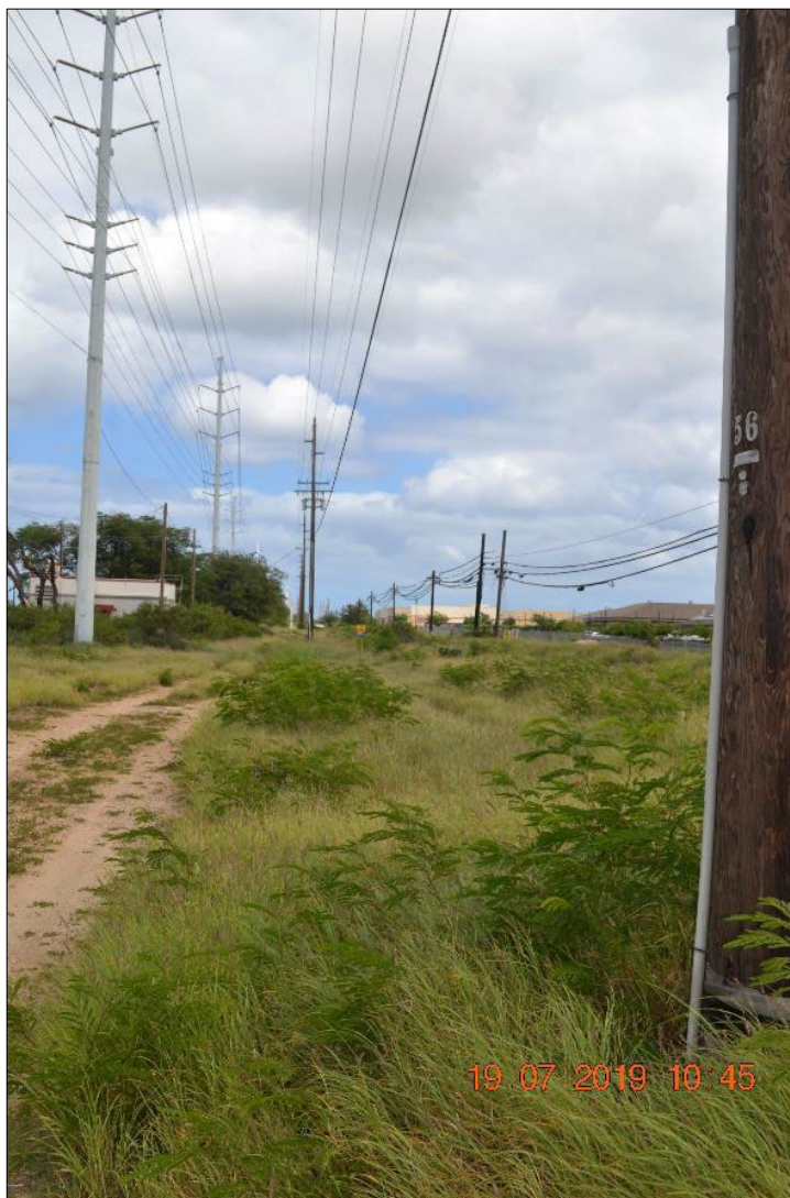
Figure 5 – Kalaeloa-Ewa Nui 138kV Circuit, CEIP-Ewa Nui 138kV Circuit, Kahe-Standard Oil 2 46kV Circuit, CEIP 46 46kV Circuit, and CEIP 3 12kV Circuit, Kapolei, Oahu 2019
