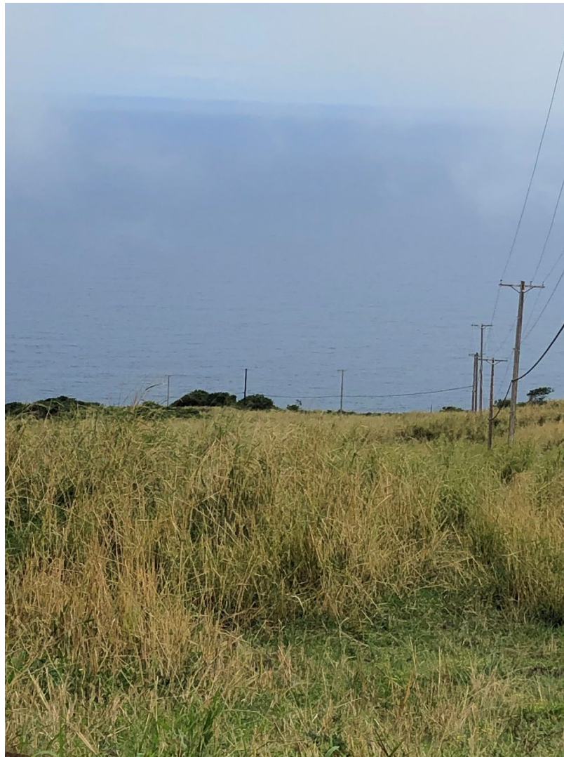
Figure 10 – Punaluu 12kV Circuit, Mauka of Honuapo Bay, Hawaii Island 2020.
